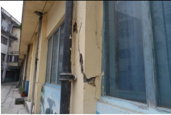
Figure 6. Cracks on Building with New ICU
