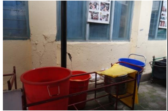
Figure 7. Cracks on building adjacent to Treatment Center
