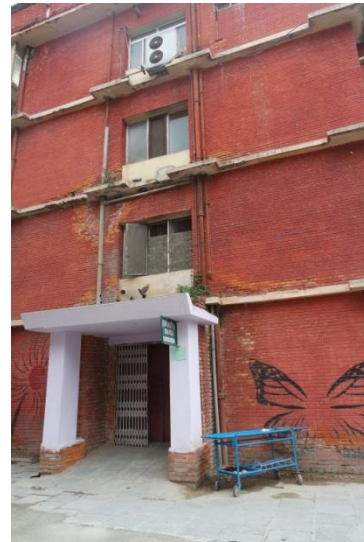
Figure 9. Old Building marked safe
