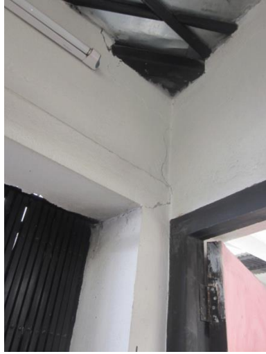
Figure 1: Cracks found in treatment center
