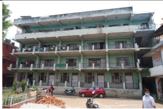
Figure 15. Building marked unsafe
