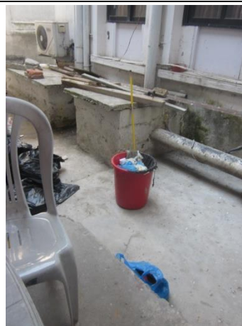
Figure 4: Misplaced bucket from ward
