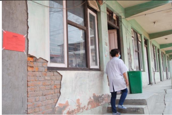
Figure 14. Building marked unsafe at Teku Hospital
