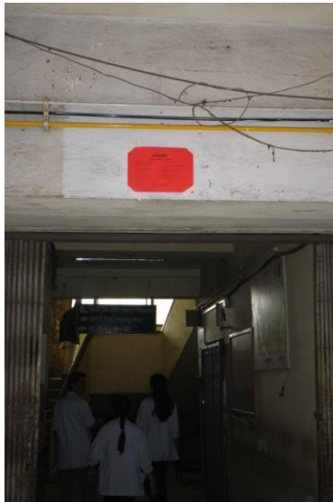
Figure 8. New ICU building marked unsafe
